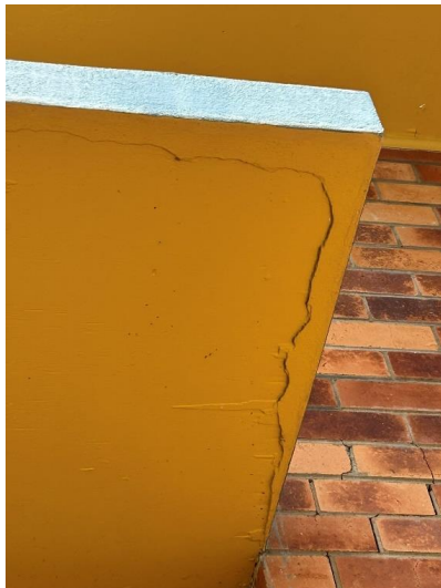
Image 31 – Cracking to Underside of Reinforced Concrete Awning
