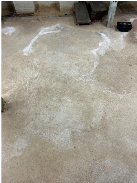
Image 12 – Efflorescence Staining to Surface of Basement Slab
