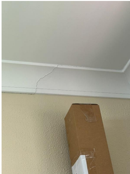
Image 26 – Cracking to Cornice
