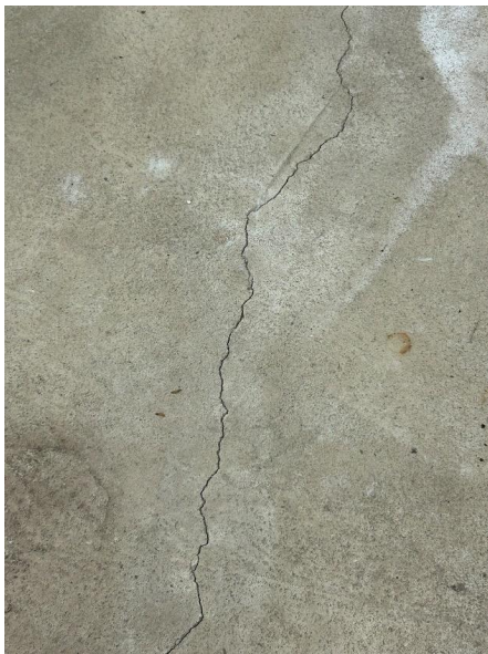
Image 11 – Cracking to Concrete Floor Slab
