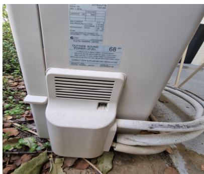
Image 13- ACU-090 Pipe Deterioration
