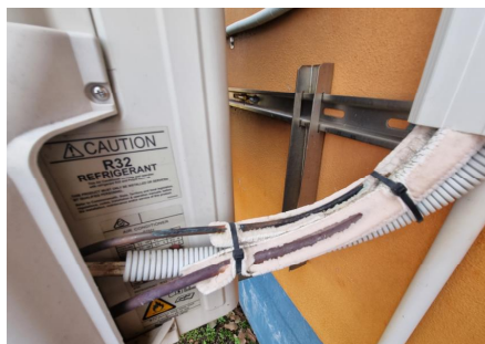
Image 15- ACU-089 pipe insulation deterioration
