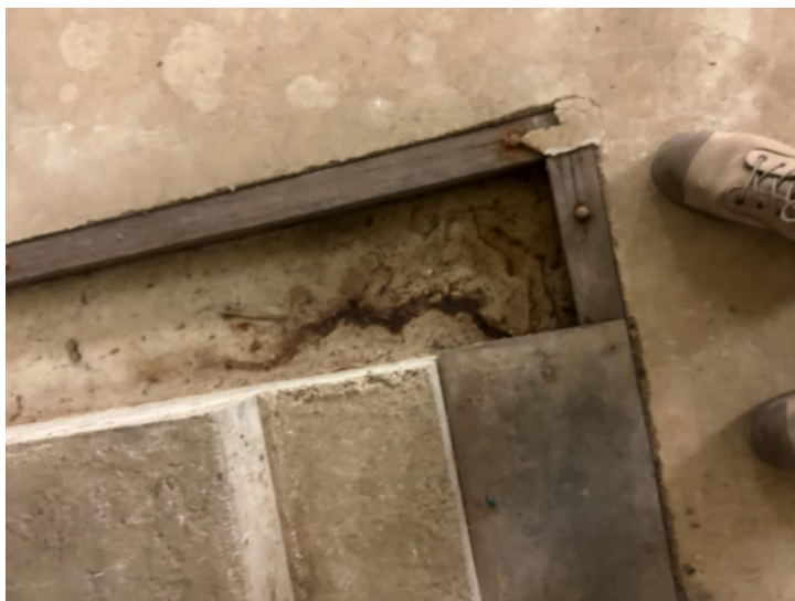
Image 13 – Moisture Staining to Existing Strip Drain.
