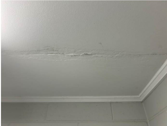
Image 18 – Ceiling Damage to Men's Toilet
