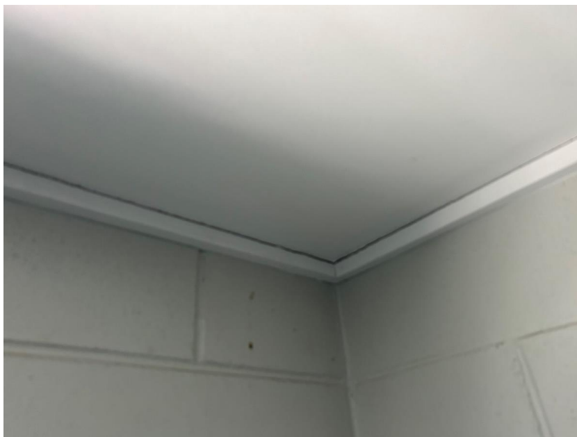
Image 21 – Gap to Cornice & Ceiling in Children's Toilet
