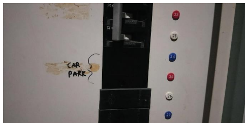
Figure 12 - Missing Pole Fillers
