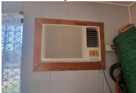
Image 4- Front Office Box/Room AC
