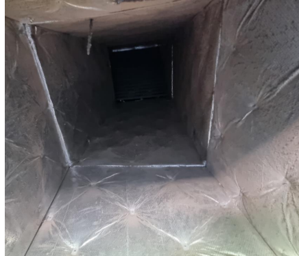
Image 8- Common Return air duct inside.
