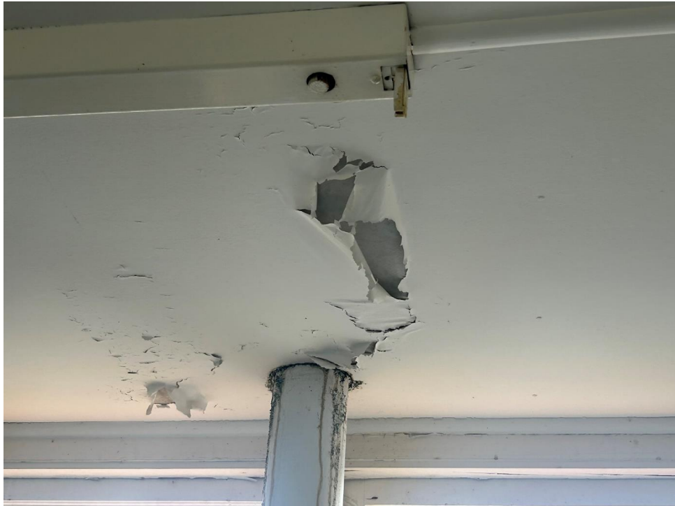
Image 36 – Ceiling Damage in Toilet
