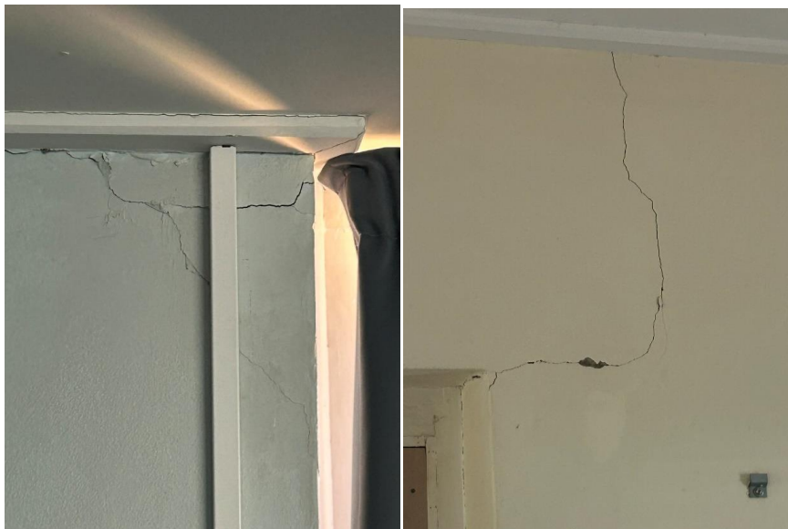
Image 34 – Examples of Cracking to Internal Wall
