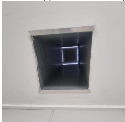
Image 10- Amenities vent blocked off
