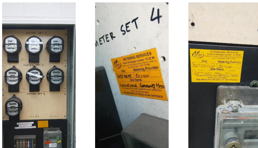
Figure 4 - Main Switchboard Metering
