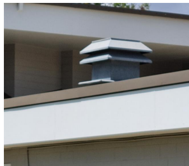
Image 1 - Roof mounted Kitchen exhaust fan
