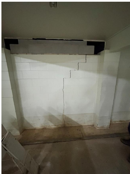
Image 7 – Cracking to Basement Retaining Wall
