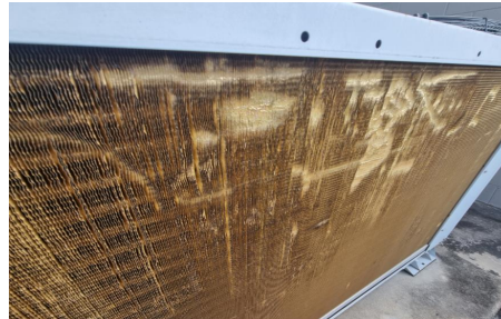
Image 6- Damaged Condenser coils
