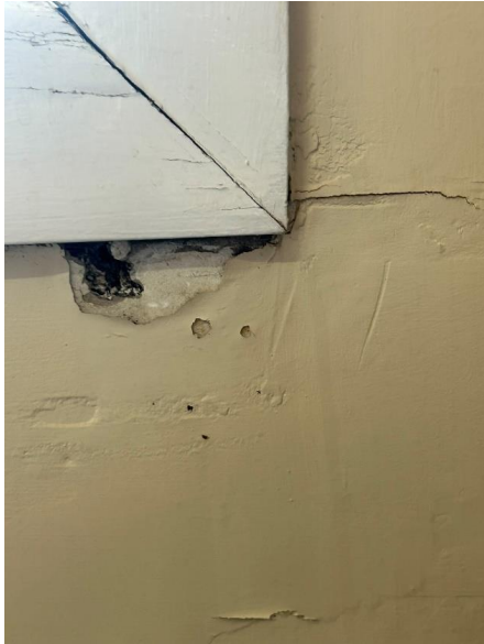
Image 28 – Moisture Damage Around Windows
