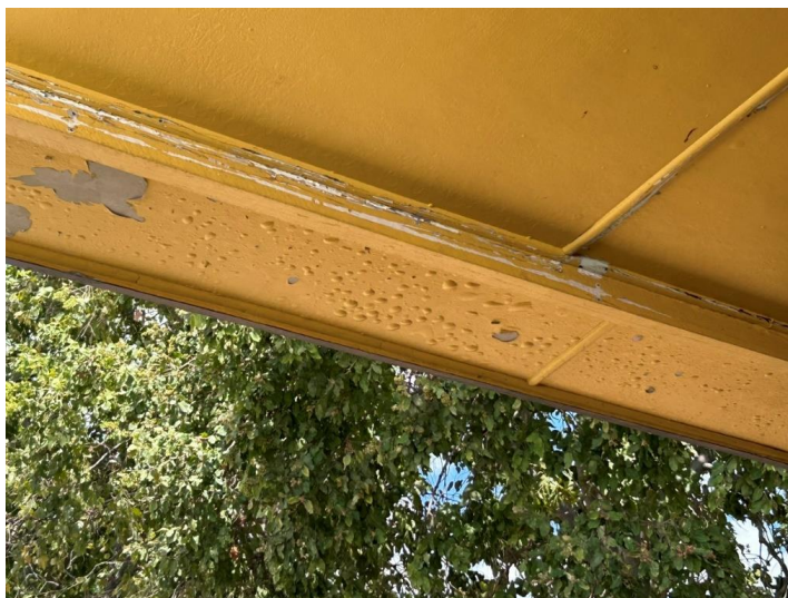
Image 32 – Bubbling to Paint on Rear Veranda
