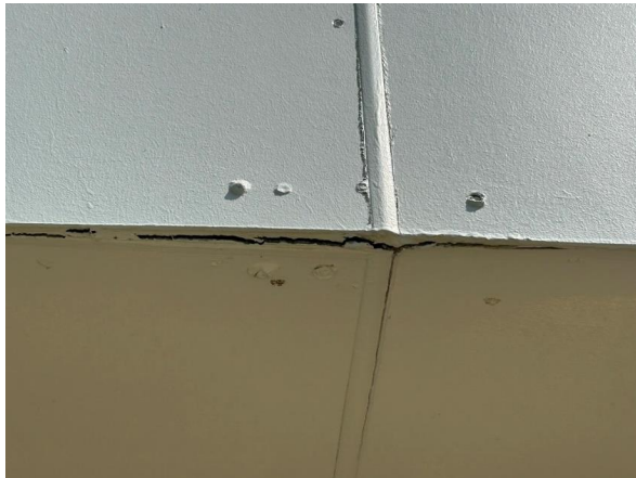
Image 22 – Damage to Parapet Cladding Adjacent Kitchenette
