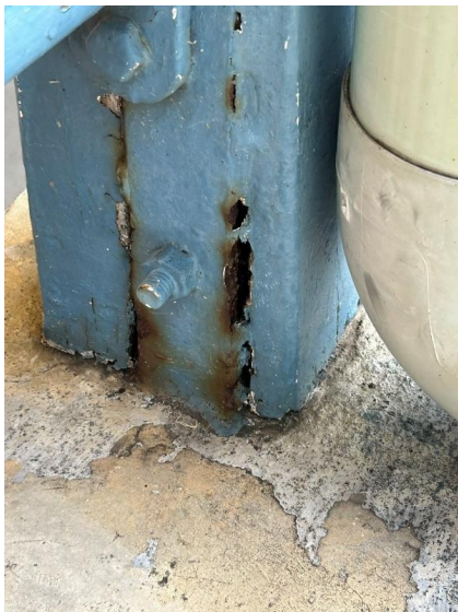
Image 29 – Damage to Base of Veranda Support Posts
