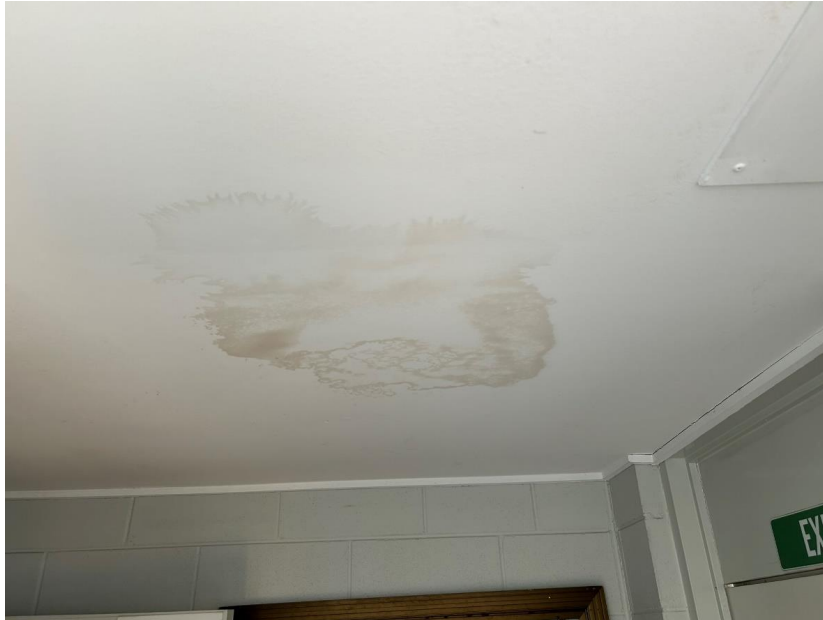
Image 20 – Staining to Ceiling at Kitchen Corridor
