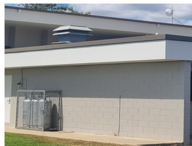
Image 6- Kitchen Exhaust Fan
