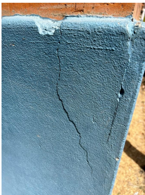
Image 33 – Cracking to Concrete Render at Corner
