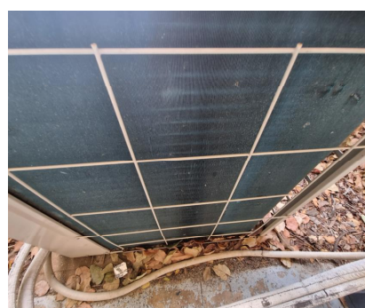
Image 14- ACU-090 Coil Condition
