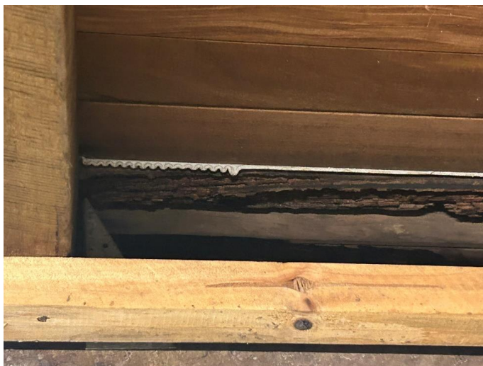
Image 9 – Rotting Timber Framing over Basement Wall
