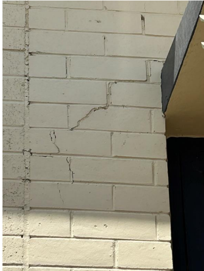
Image 24 – Cracking to External Brickwork
