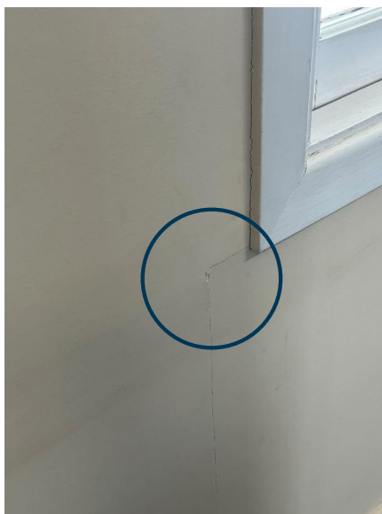
Image 27 – Cracking to Inside Face of Brickwork
