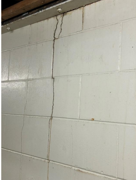
Image 10 – Tannin Staining to Face of Block Wall
