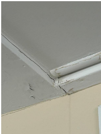
Image 25 – Moisture Damage to Ceiling
