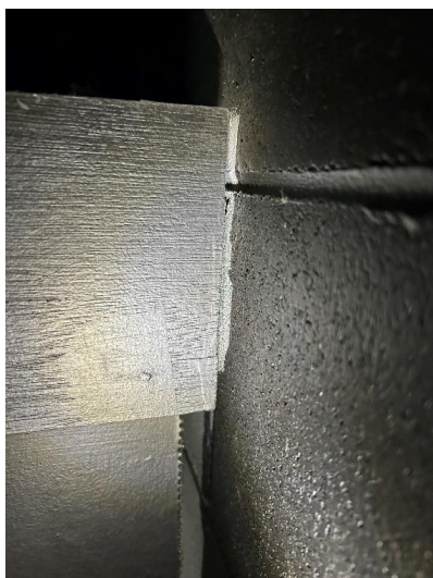
Image 17 – Gap Between Internal Stud Wall & Perimeter Block Wall
