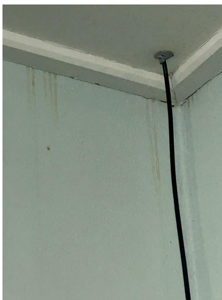
Image 35 – Example of Moisture Staining to Walls
