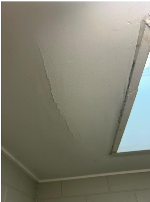
Image 19 – Ceiling Damage to Woman's Toilet
