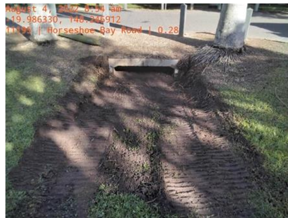
Horseshoe Bay Road – Unblocked Drain Outlet
