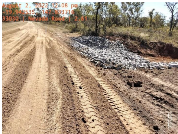
Nevada Road – Scour repair on shoulder
