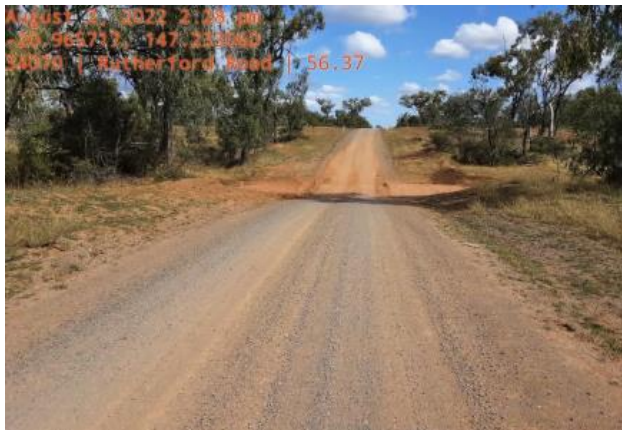
Rutherford Road – Clear sand and silt build up
