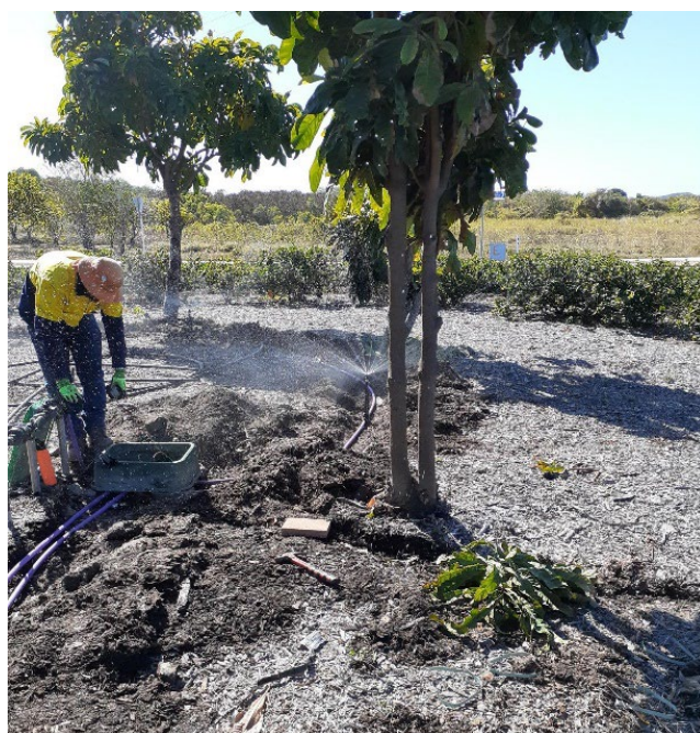
Hay Street round-a-bout irrigation installation.
