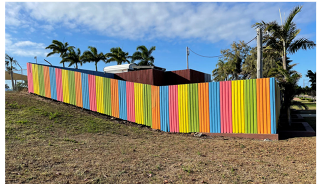
Photo 6: Painted Fence - Bowen Swimming Pool
