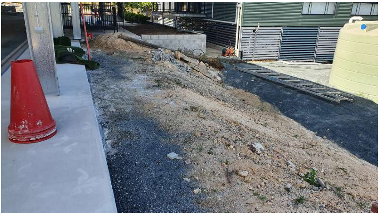
Unusable and unsafe area left after Rainwater Tank Project
